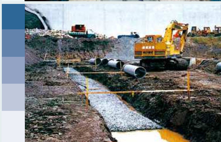
集水管 Water collecting pipes
