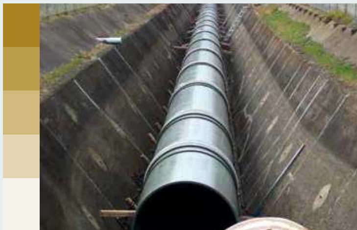
農業用水管 Agricultural Water pipes
